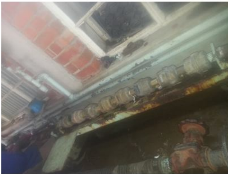
Meter testing in progress
