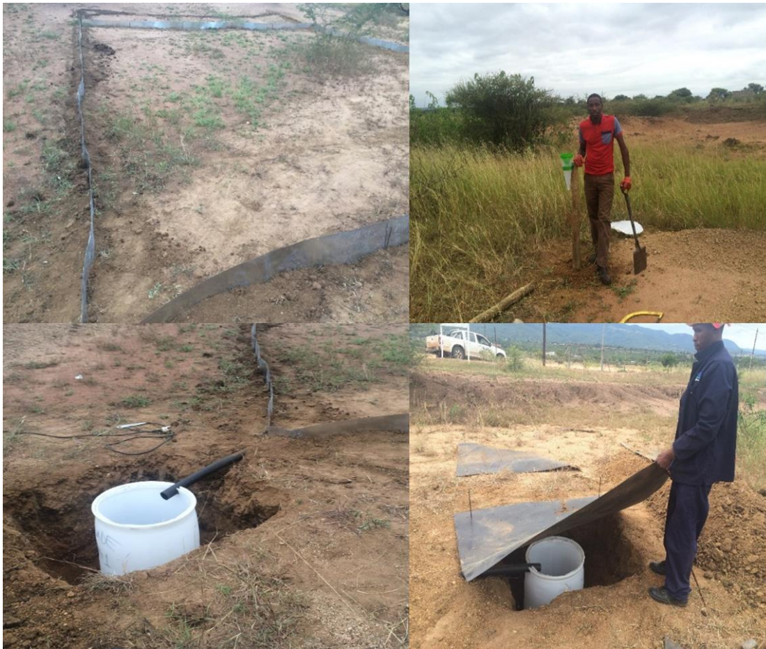
Figure 4-3: Installation of the runoff plots (top-left), Rain gauge (top-right), Sediment collector (bottom-left) and cover to prevent direct rainfall (bottom-right). (Images taken on 6 January 2016)
